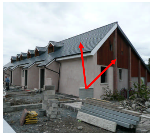
Fig. 5 : Omitted dormer and new openings in the western elevation
